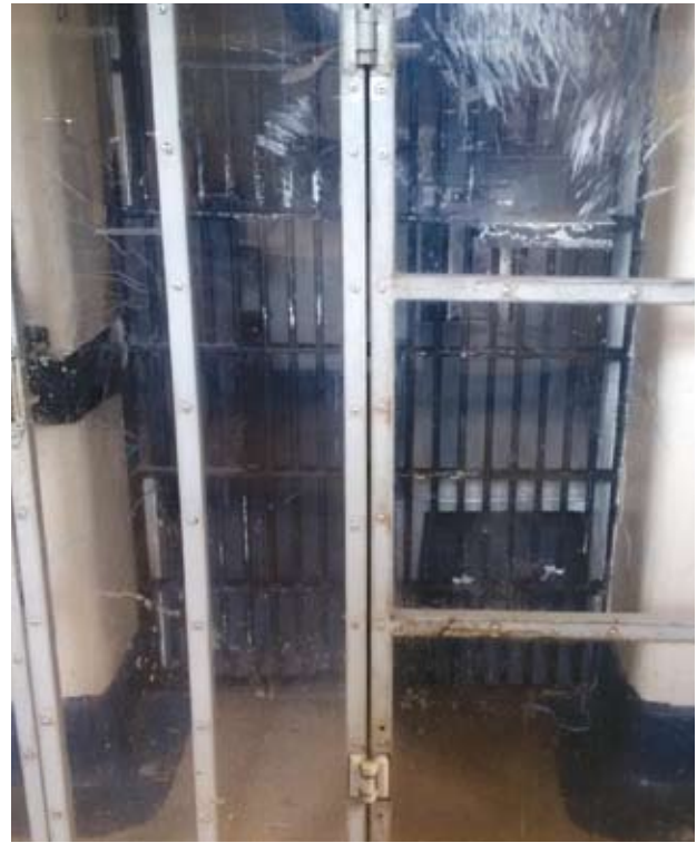
Segregation cell covered over in plastic safety glass
